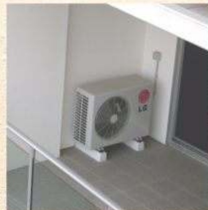
Dedicated Space for A/c Outdoor Units.
